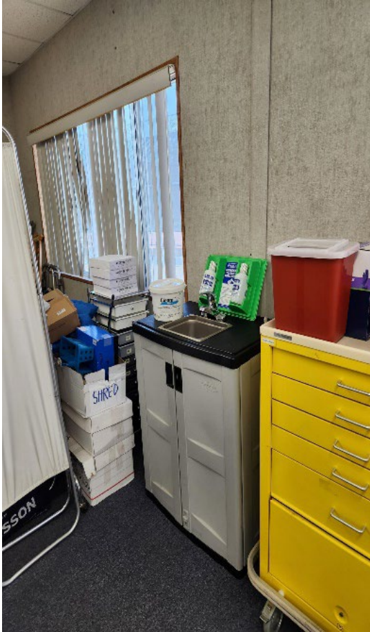
Sink without plumbing
